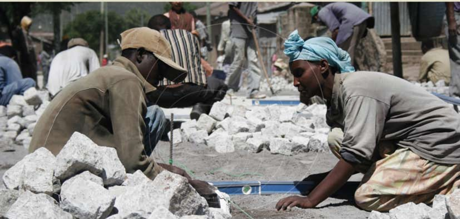
Pavers in Adama have already laid over 50,000 square meters of Cobblestone roads.
